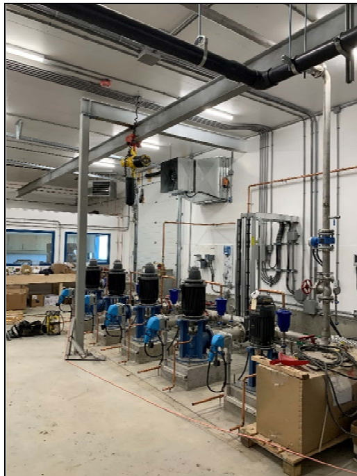
Distribution pump lineup with all electrical wiring and connections completed.
