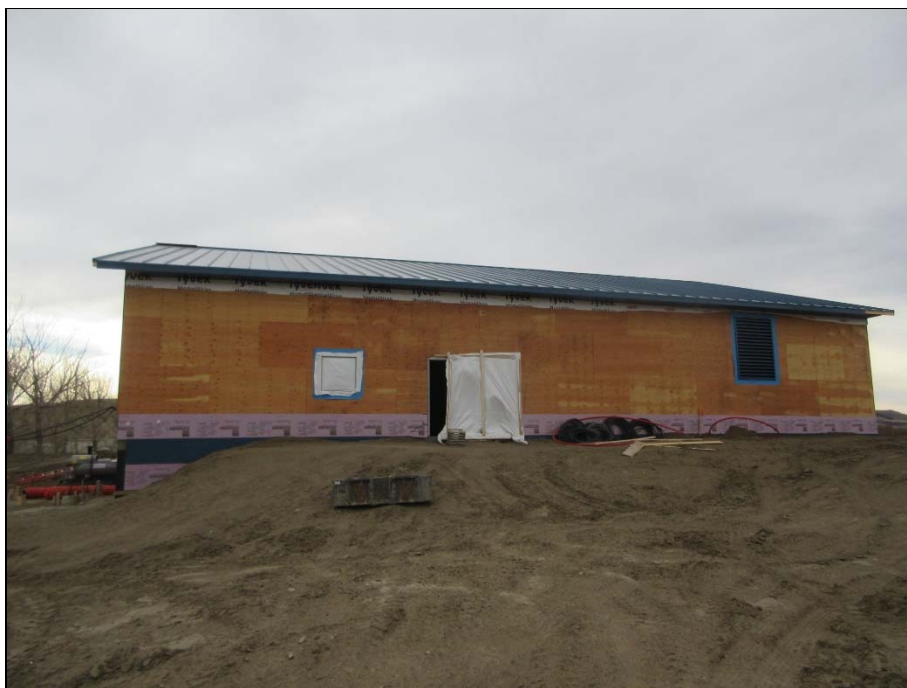
Front of water treatment plant – compaction completed except at left around the proposed loading dock and retaining wall location.
