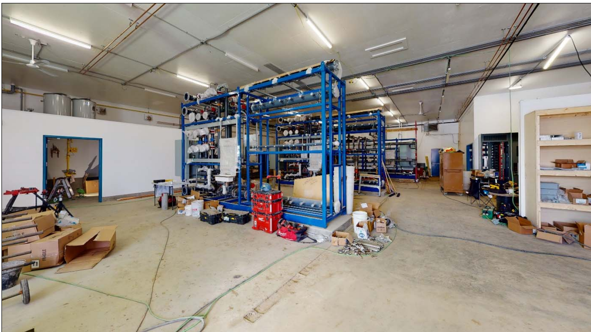
Treatment skids are installed; domestic water piping and electrical conduit installation started.
