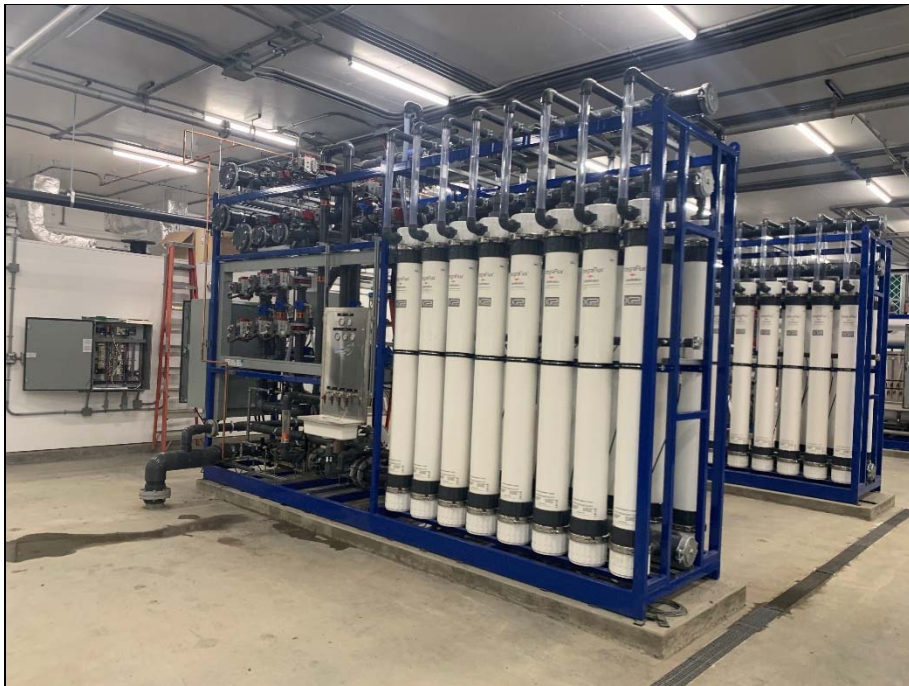
Ultrafiltration membranes (white vessels) are now loaded up and starting to filter water.
