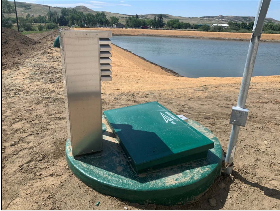
Effluent pumping station.
