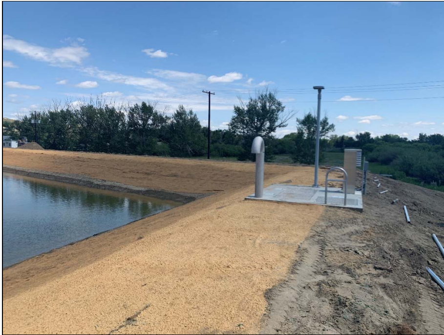
River intake pumping station.
