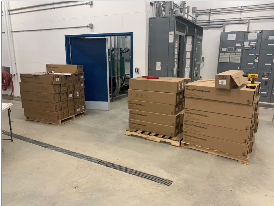
Nanofiltration membranes on site and ready to be loaded (have since been installed).
