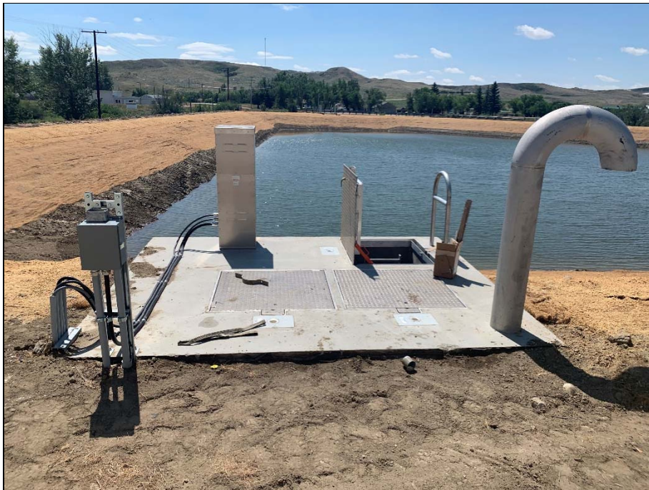
Reservoir intake pumping station.
