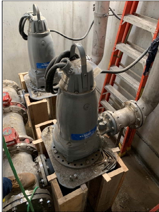
Intake pumps and piping.
