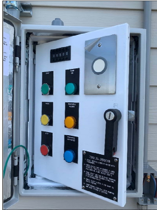
Truck fill control panel.
