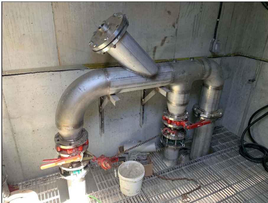
Intake pumphouse piping and valves.
