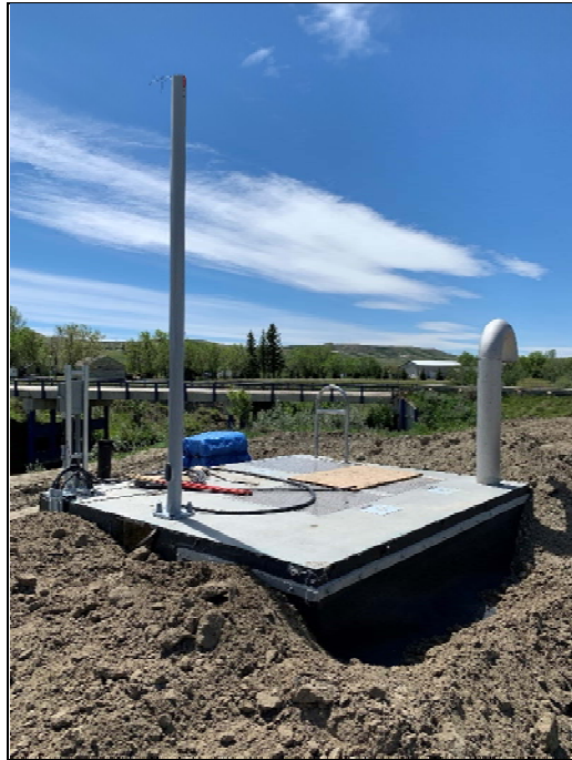
River intake pumphouse.
