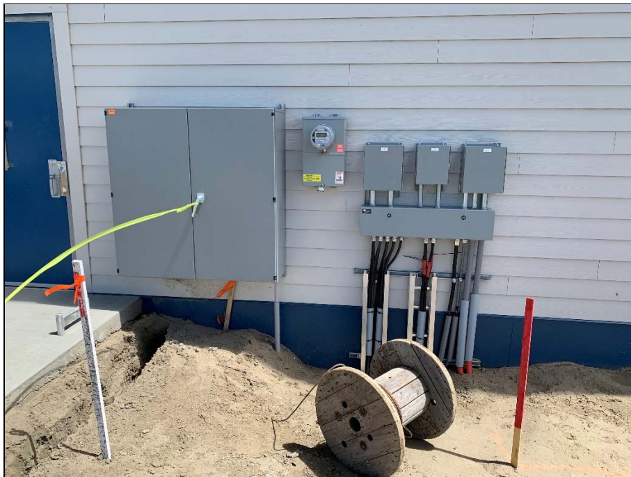
Electrical service area – 600V, 120V and 24V junction boxes.
