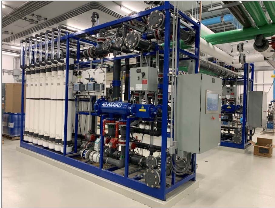
Ultrafiltration system skids – floor and curbs epoxy painted.
