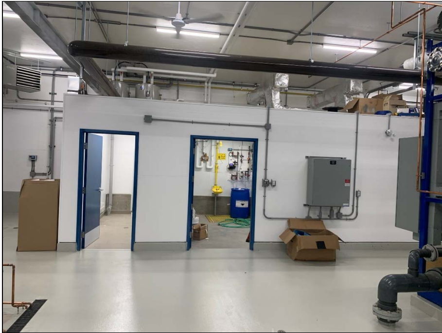
Washroom and chemical room entry areas cleaned up and floor epoxy completed.
