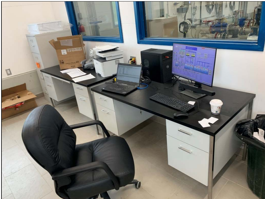
Office furniture is now set up and will be cleaned up following commissioning.
