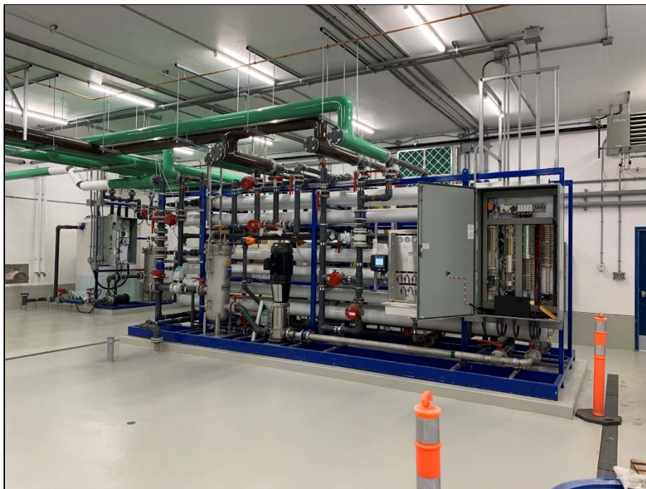
Nanofiltration skid; PLC wiring / program checks underway.
