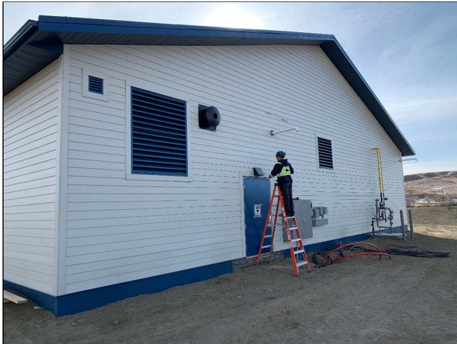
West side siding is complete and electrical and gas service equipment in place.
