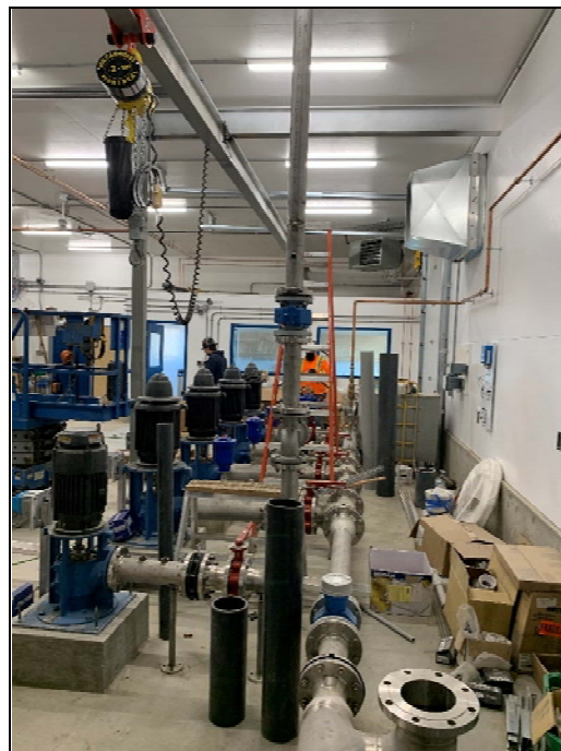
Distribution and truck fill piping.
