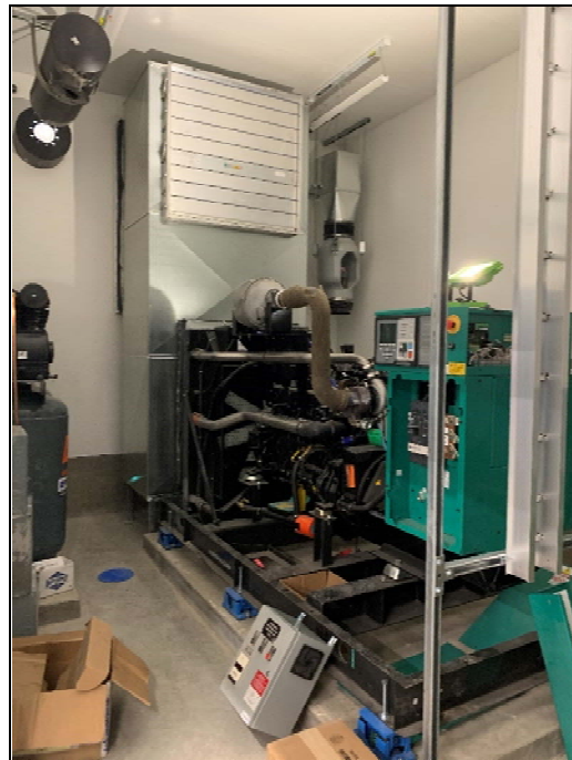
Generator and ducting in place.
