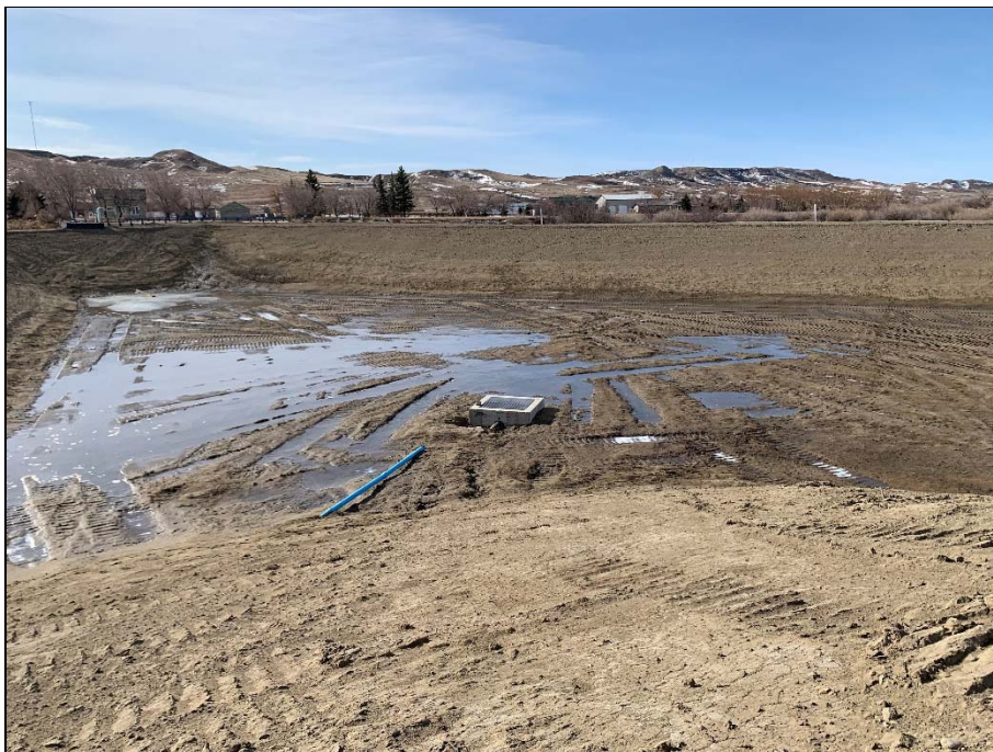
Reservoir floor is starting to dry up; once dry the construction and liner work can resume.
