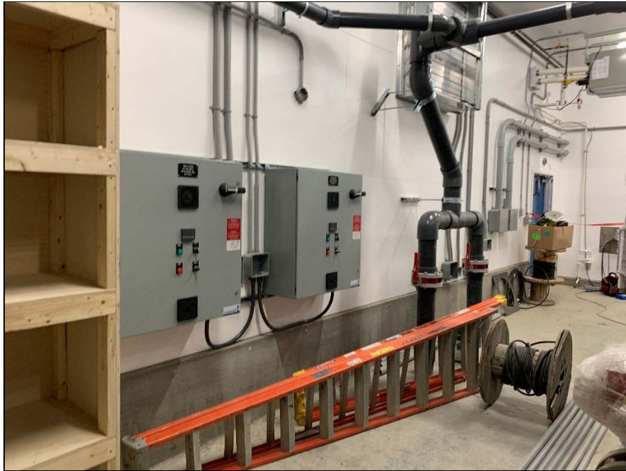
Wiring and control panels located throughout the building.
