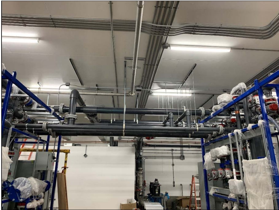
Electrical wiring and conduit runs.
