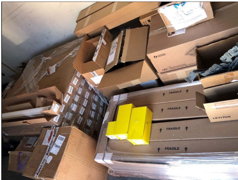
Additional electrical material on site.
