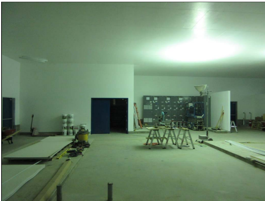
Generator room painted and doors in place; motor control sections.
