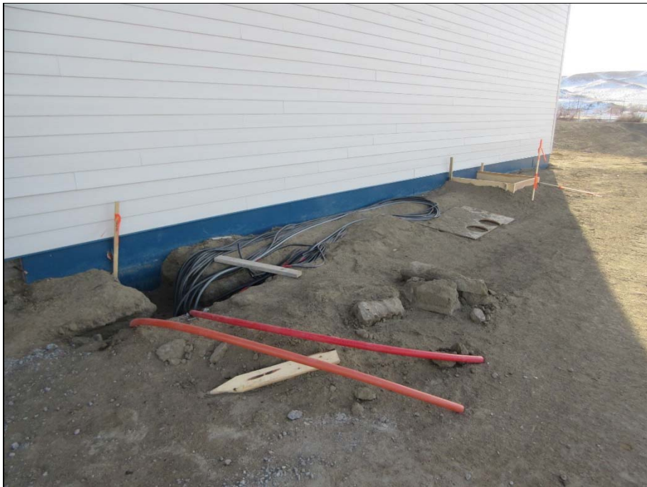
Electrical lines from raw water pumping stations relocated to west side of plant.
